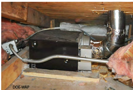
Right-way fan orientation: Air stream turns 90 degrees which is acceptable.
